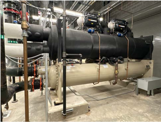
FIGURE 2: DAIKIN WATER-COOLED CHILLER
