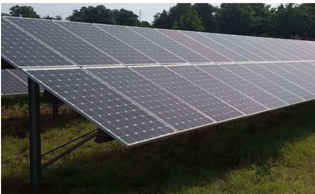
FIGURE 4: ON-SITE POWER GENERATION
